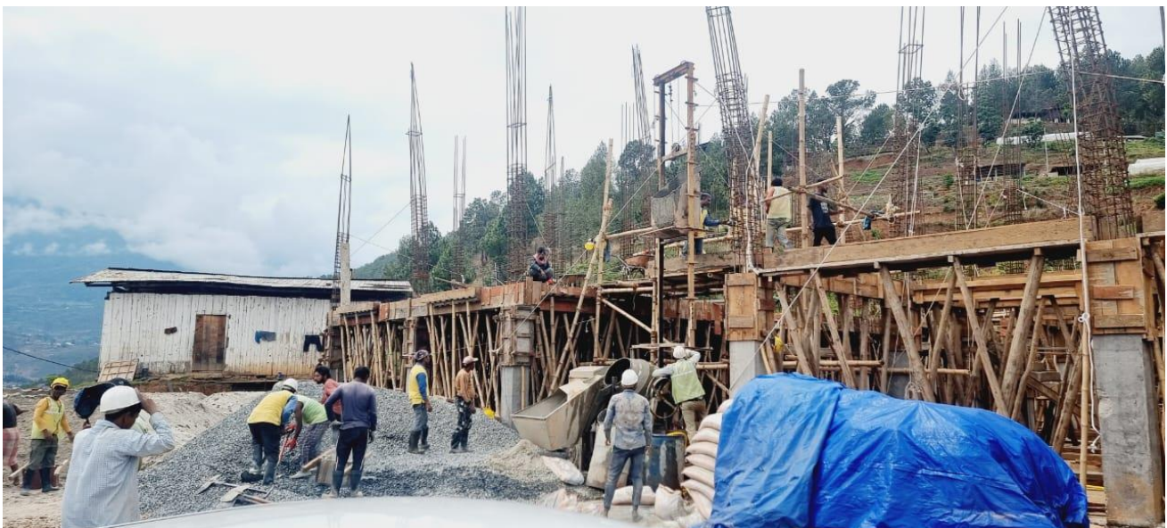
Fig. 7: Workers without PPE
