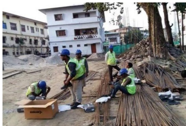
Few workers found using PPEs during inspection
